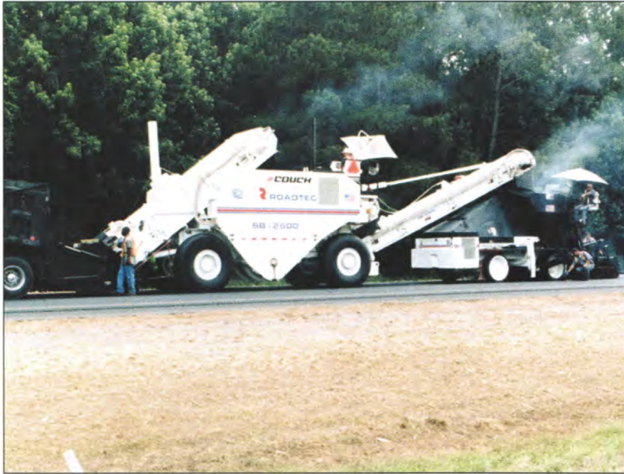
The material transfer device used on the I-10 project remixed the stiff mix and enabled the paving train to keep moving, producing a smooth pavement.
