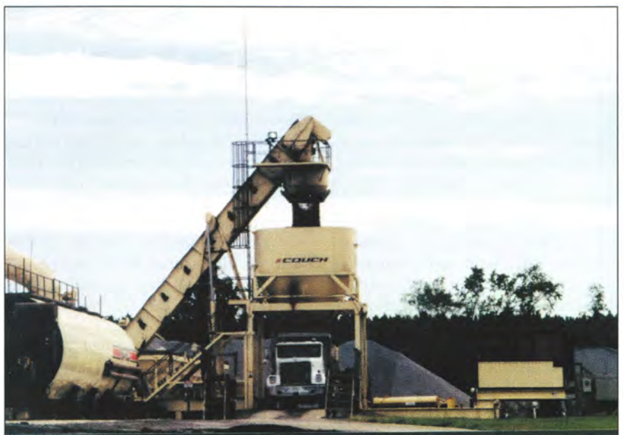
The purchase of a new asphalt plant for use on the project allowed plant operators to make minute adjustments to the mix and achieve the proper amount of air voids.
